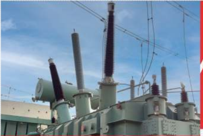
RIP Bushing installed on a transformer as a replacement to existing OIP Bushing in Y phase with R&B phase operating with the old OIP bushing
